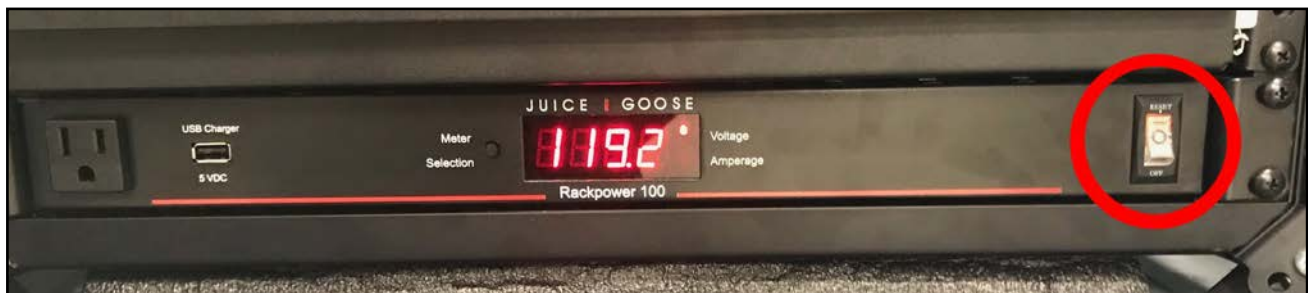
AC Power Distribution Unit Switch
