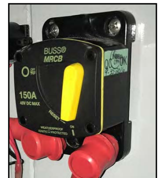
Battery Breaker (On Position)
