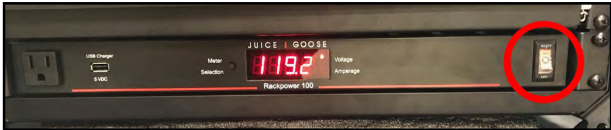
Figure 38: AC Power Distribution Unit Switch
