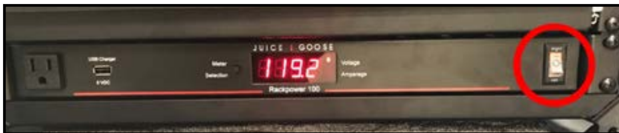
Figure 37: AC Power Distribution Unit Switch
