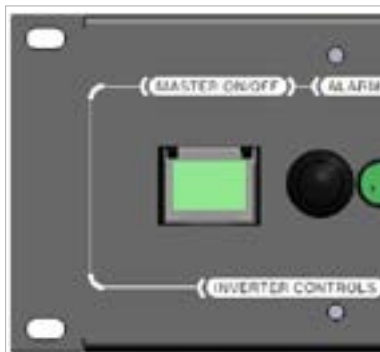
Figure 14: Patch Panel Master On/Off Switch
